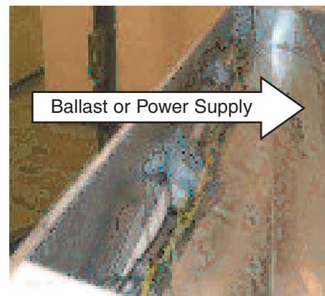
Ballast or Power Supply Location
