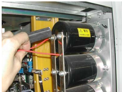
Picture 5-3 rectifiers filters turn on electricity of an electrolysis electric capacity
