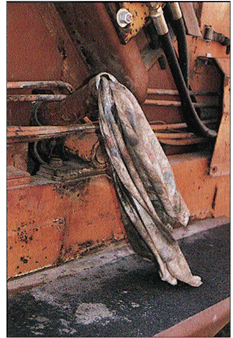
Dirt is the number one enemy of hydraulic systems. Ineffective practices—such as using a rag in place of a lost or misplaced filler cap on this hydraulic reservoir filler spout—allow dirt to enter the system and destroy valuable components.
