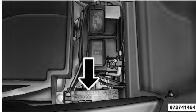
Rear Power Distribution Center
