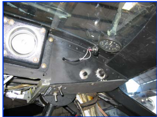
MASTER AIR CONDITIONING CONTROLS & FORWARD FAN SPEED CONTROL SWITCHES (OVER PILOTS HEAD TO RIGHT OF THROTTLE)
