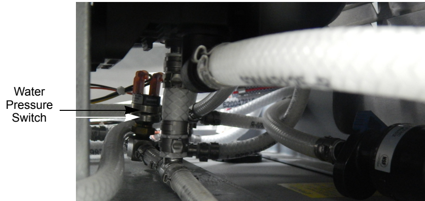
Figure 49. View of Water Pressure Switch
