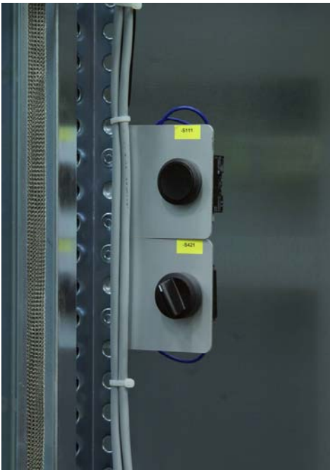
Figure 3-3 Fast ON button and local/remote selector switch
