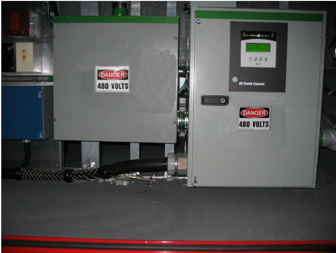
Figure 24: ATS Control Panel
