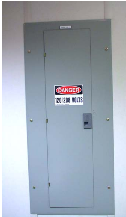
Control Room Panel
