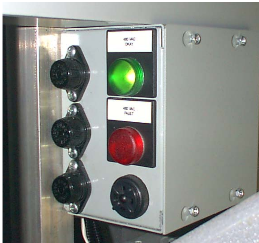
Figure 62: 480V AC Phase Power Monitor
