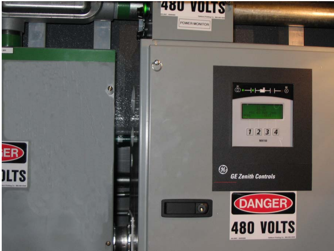
Figure 61: 480V AC ATS and Phase Power Monitor
