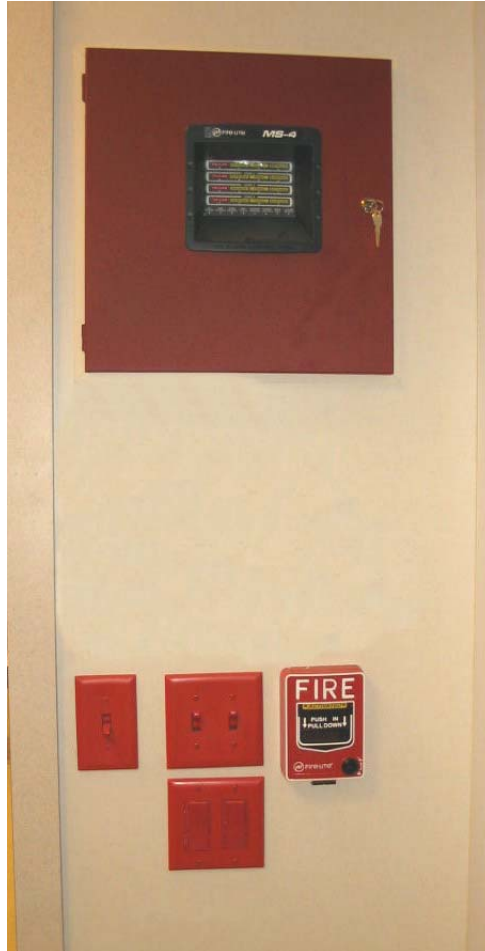
Figure 10: Control Room Controls
