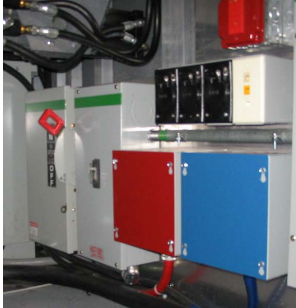
Figure 36: Fire Alarm and Code Blue Alarm Junction Boxes
