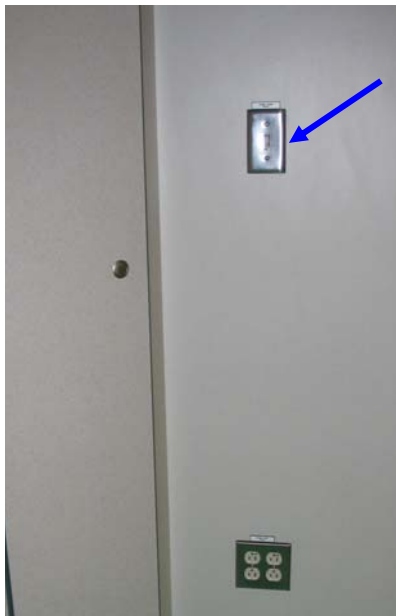
Figure 63: Power Receptacle/Light/Light Switch
