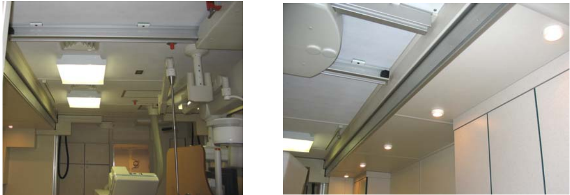
Figure 79: Procedure Room Lighting
