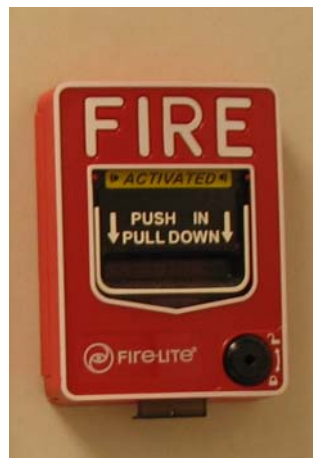
Figure 35: Fire Suppression Pull Station
