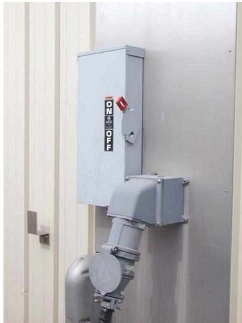
Figure 59: Shore Power Connection
