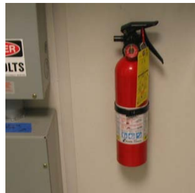
Equipment room location
