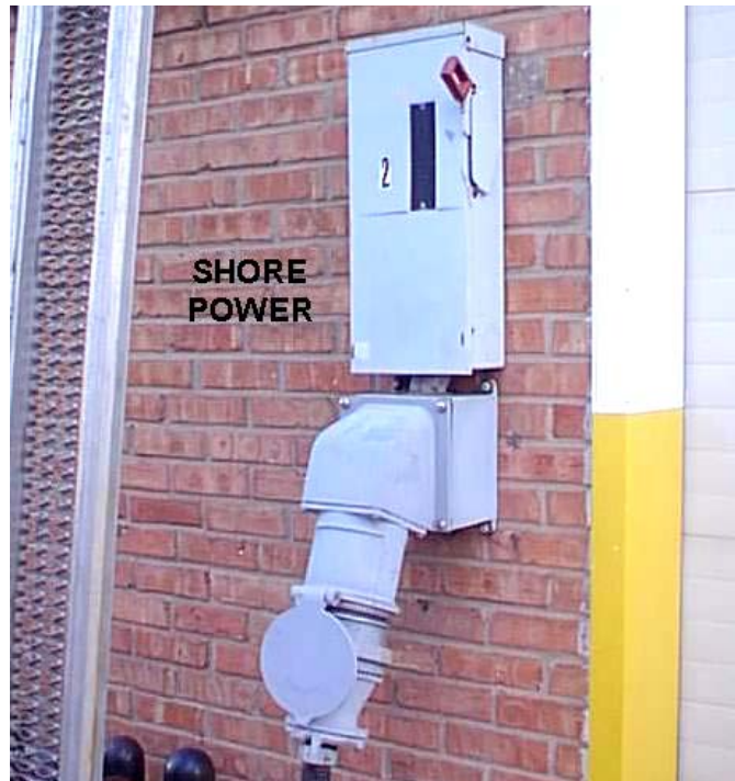
Figure 8: Shore Power Connection.
