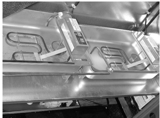
Condensate Pans; Primary (left) & overflow (right)
