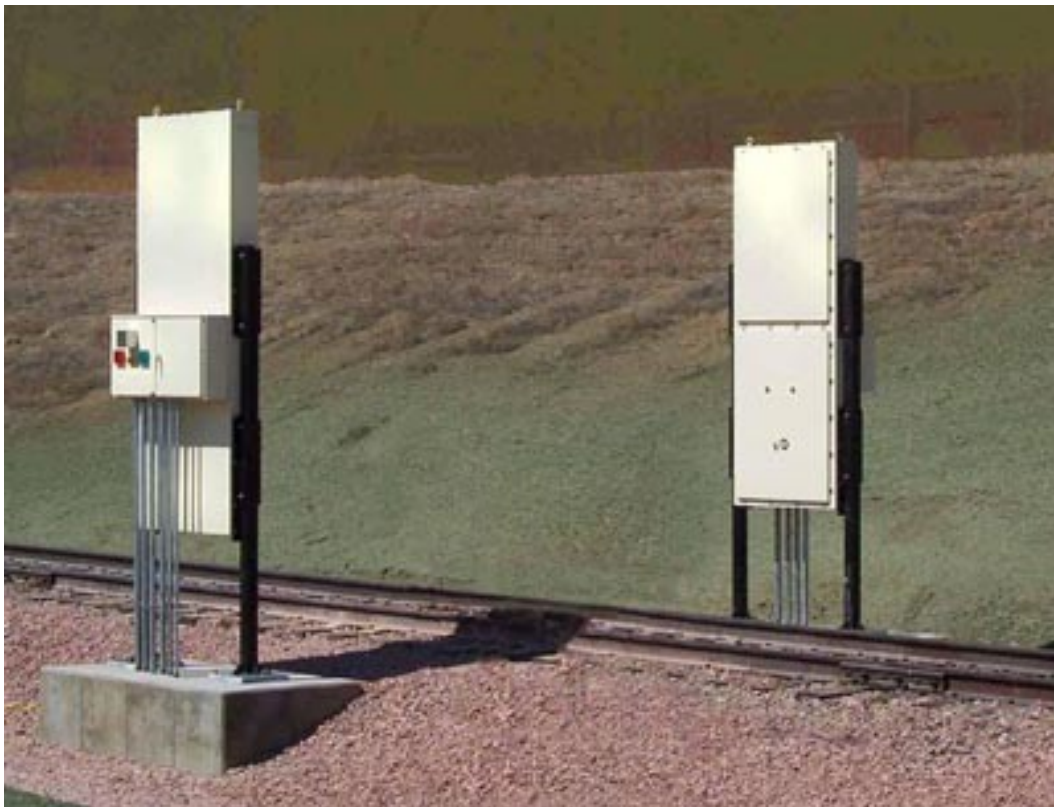
TM-850 in a railroad monitoring application ( the electronics box on the back can also be mounted on the bottom)
