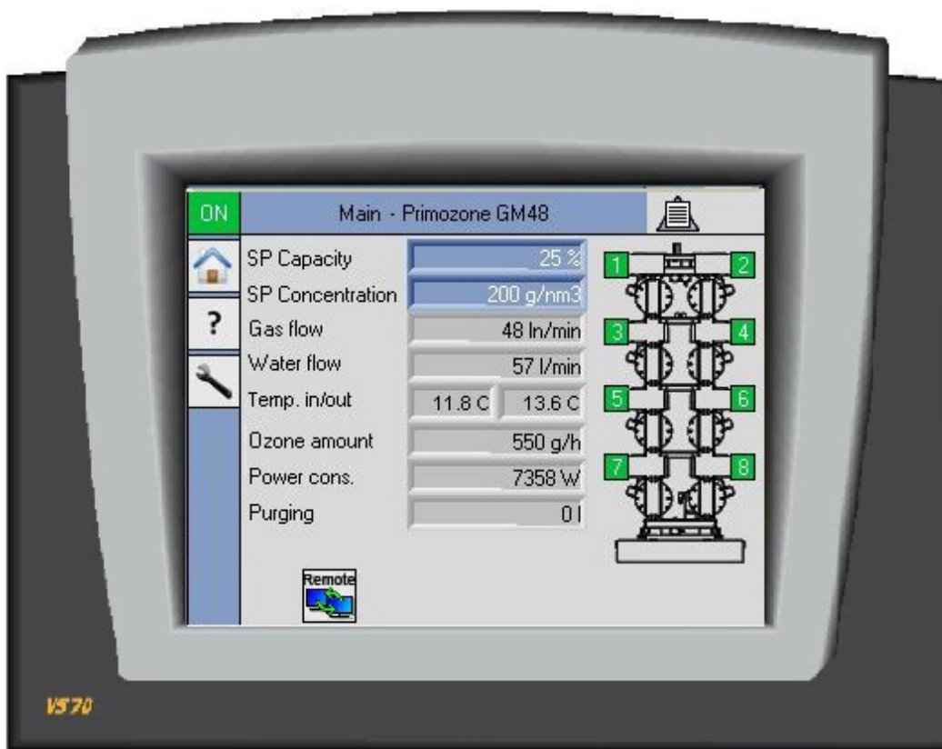
Figure 7, Showing the LOCAL/REMOTE HMI on Primozone GM48
