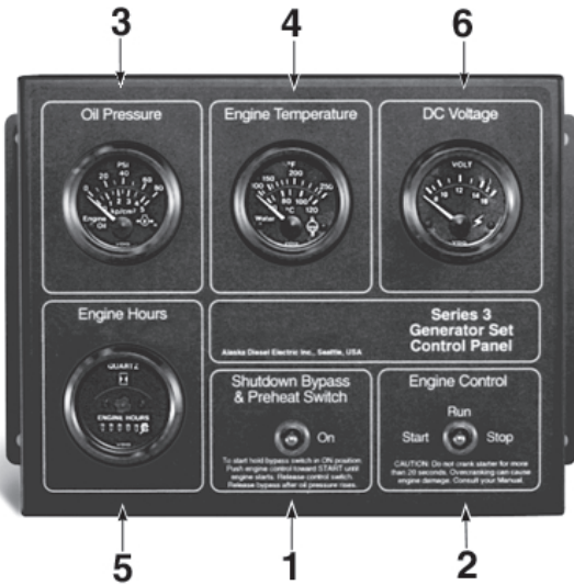
Figure 3: Series 3 Generator Control Panel
