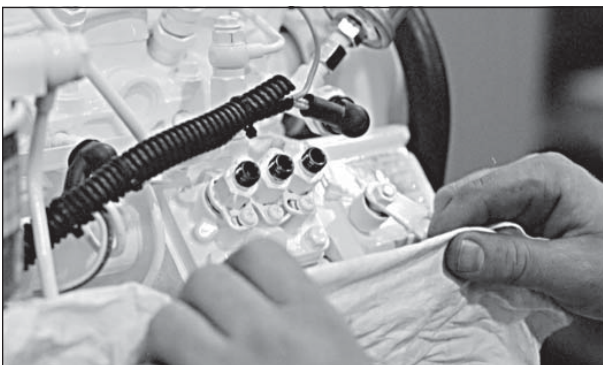
Figure 14: Cover lines, inlets and injection pump outlets.
