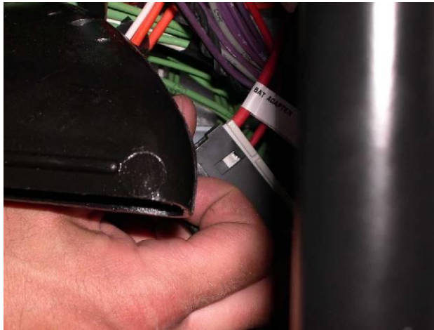
Figure 11 - Battery (red) splice pack
