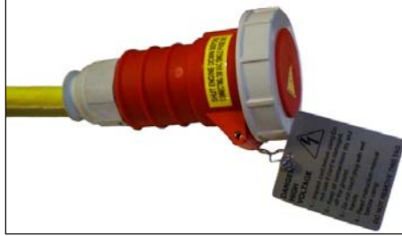
Figure 11: Power-supply receptacle with warning tag.
