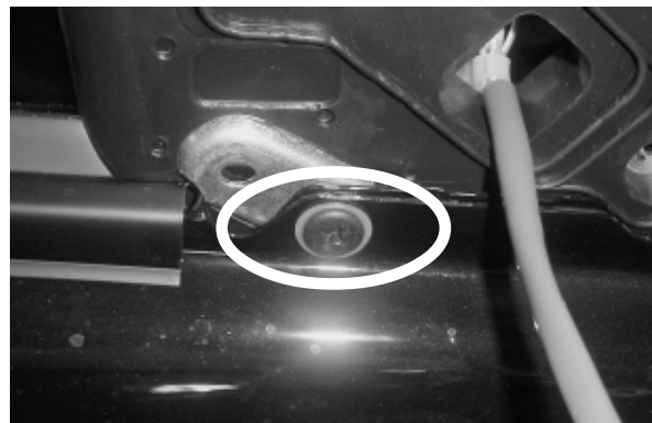
Below: The Gusset screw that causes the circuit to short out.
