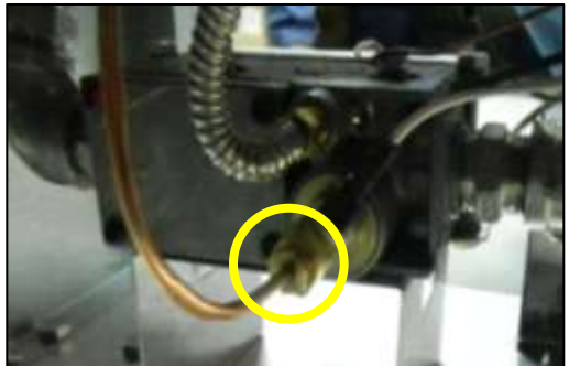
Disconnect thermocouple from the combination valve
