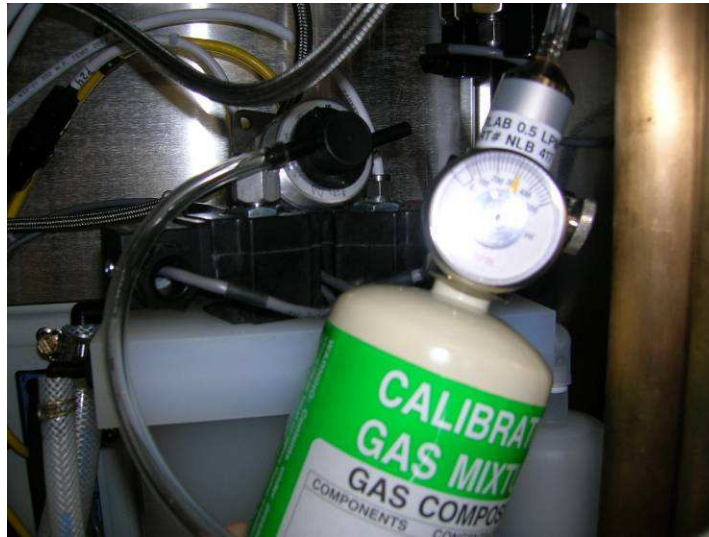
Figure 17 Calibration Hood installed on Combustible Gas Sensor
