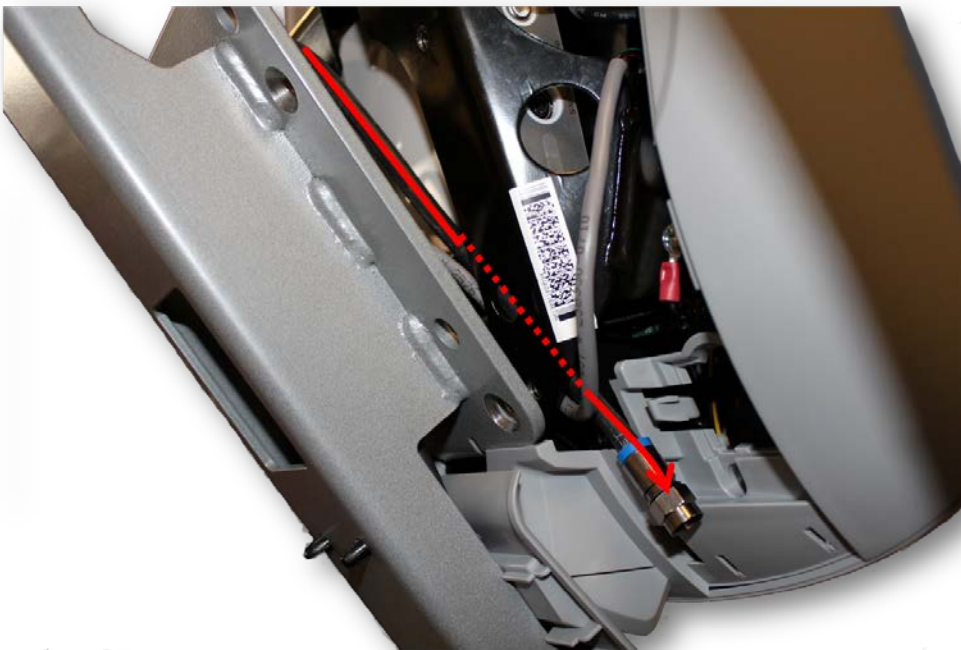
Figure 4: Coax Cable Starting Path
