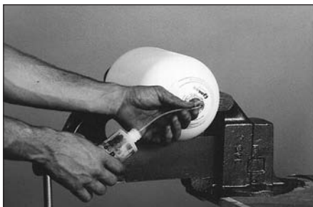
14. Using a charging and gauging assembly, precharge to the desired pressure at a moderate rate, using DRY NITROGEN only. Check the valve for leaks with snoop or soap water.
