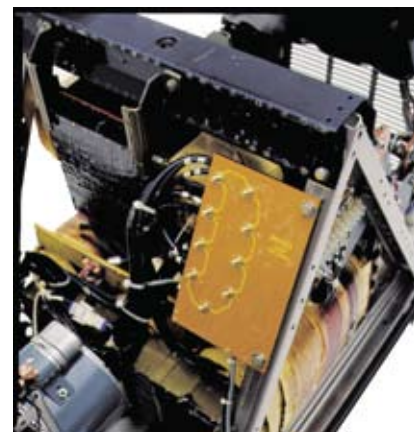
Coated Power Components & Panels
