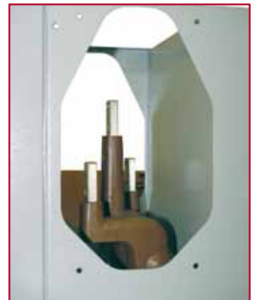
Mk II busbar chamber
