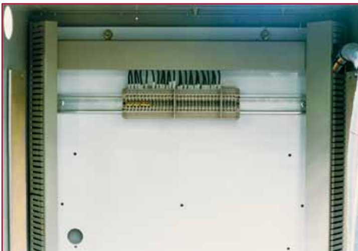
Control & Indication Cable Terminal Blocks
