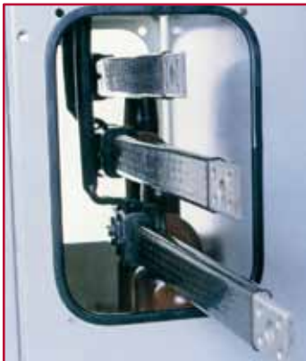
Mk 1 Busbar chamber with interconnecting busbars and associated busbar shrouds in position. Busbar connected VT risers can also be seen.
