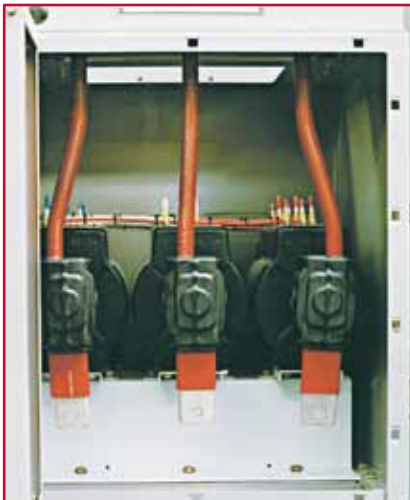
Single cable box with circuit connected voltage transformer housing fitted. (Covers removed to show internal details.)
