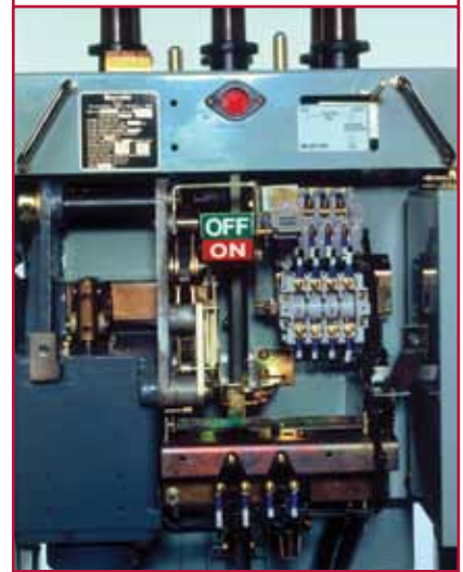
Solenoid closing mechanism – cover removed. (Type MO, X Series circuit-breaker.)
