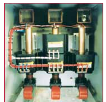
Current transformer chamber top view
