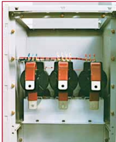
Single Cable box without voltage transformer. (Covers removed to show internal details.)
