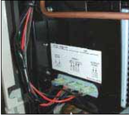
Battery for back-up
