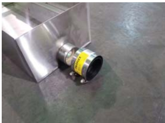
Showing the scrap box rear exit drain hub connection
