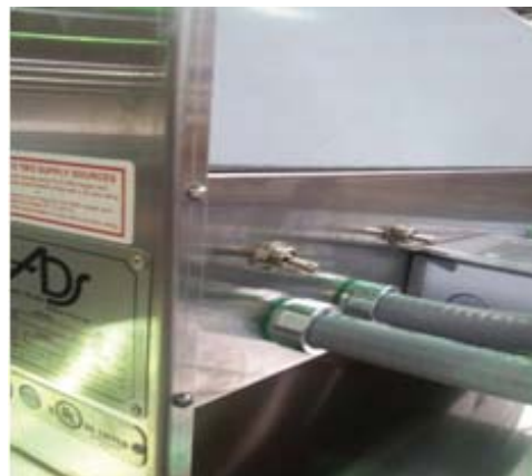
Showing the two master switches
