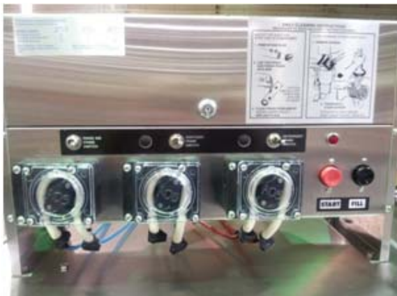
Showing the control box with chemical pumps, prime switches, red start and black fill switch
