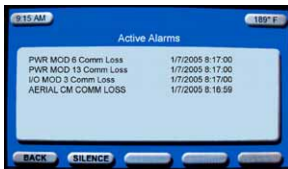
Figure 3-41: Active Alarms Screen
