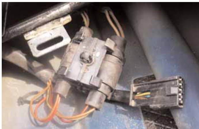
Photo #2 Connectors Inside Door
