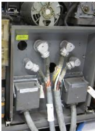
Figure 35: Power and Signal Cables in the 1402
