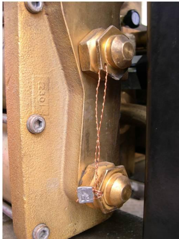
Typical Sealing of the Mechanical Calibration Device on the Flowmeter
