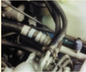
Fuel Filters and Hoses
