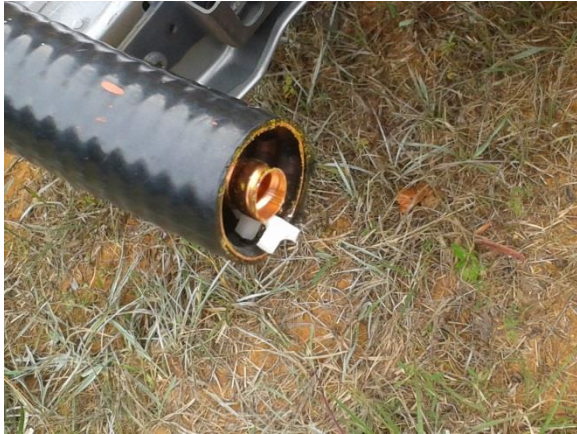
Figure 3 - Part of the old coax section, obviously damaged by water.
