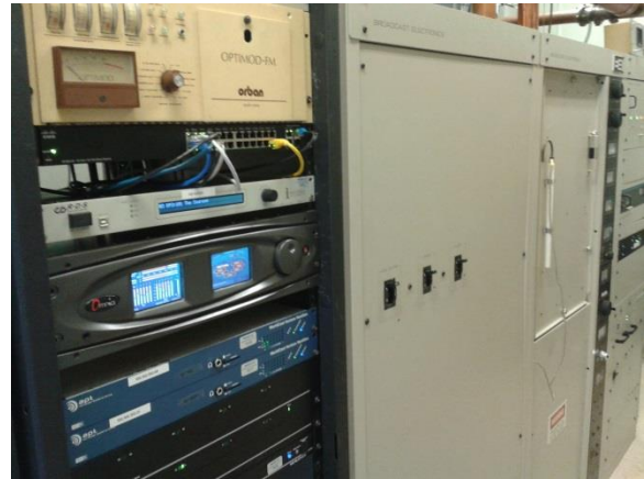
Figure 2 - The old Optimod filling a hole formerly occupied by an Intraplex.
