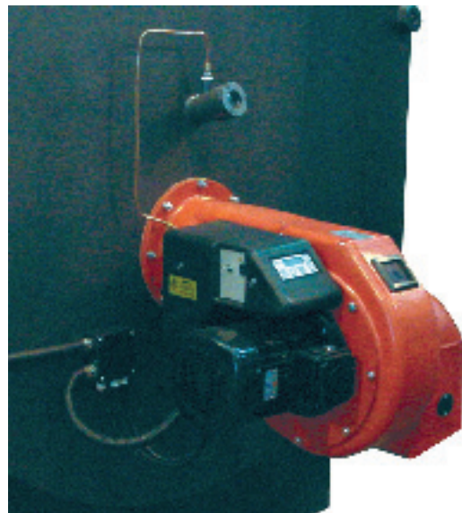
FIG. 10 OIL BURNER INSTALLATION (installation will change with the type of burner fitted)
