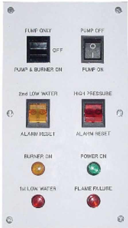
FIG. 15 BOILER CONTROL PANEL
