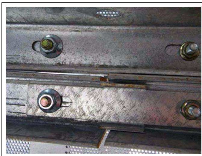
Figure 10N Gap Un-Caulked
