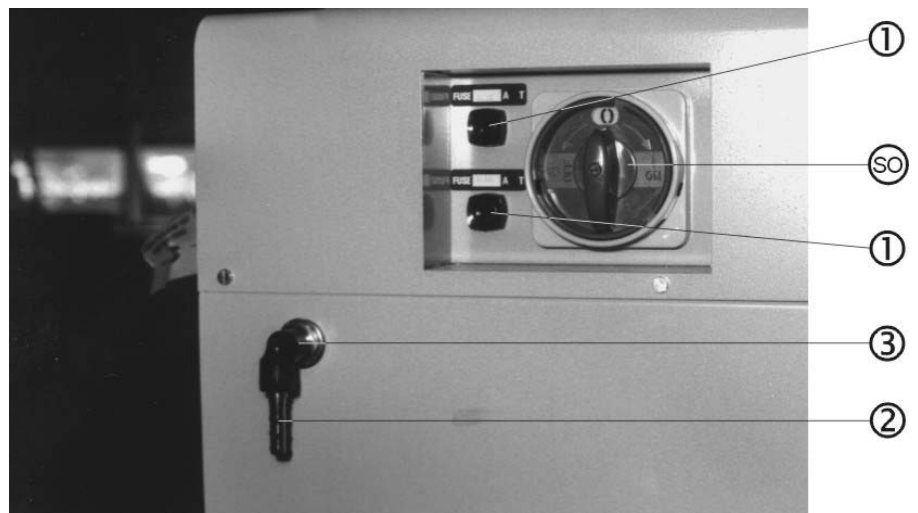
Fig. 32 Main Switch and Fuses
