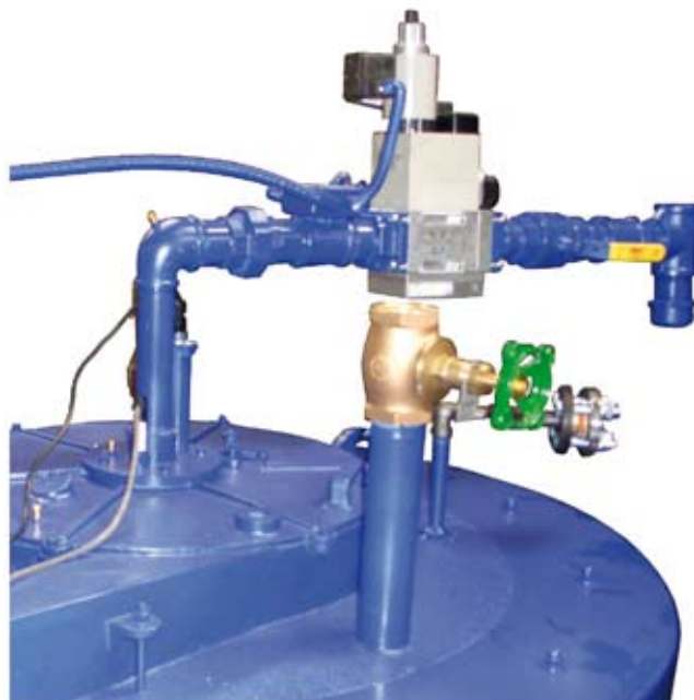
FIG. 7 MAIN STEAM VALVE
