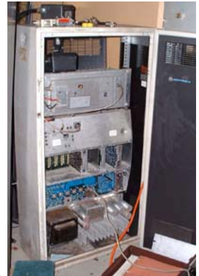
Motorola Micor repeater being transformed into the new PCARA 2m repeater at N2CBH.
