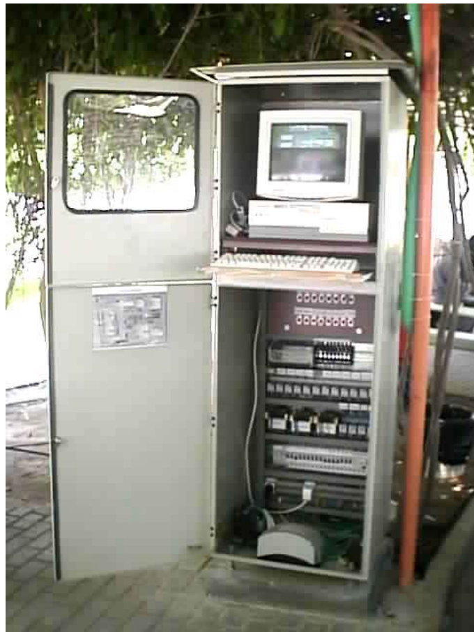
Figure 9. The implemented electric board.
