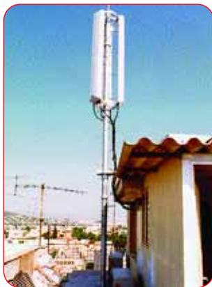
Base station in urban area
