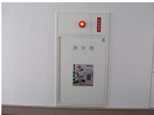
Indoor fire hydrant
