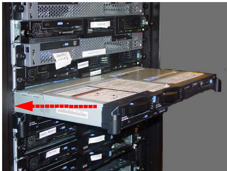
Figure 12: Slide the server into the rack
