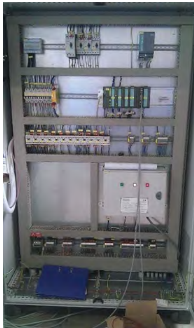
Inside View Electrical Cabinet
