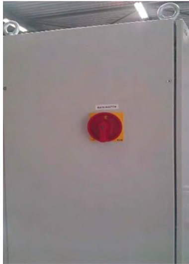
Main Power Switch
