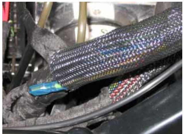
Slide the mesh back over the loom and the completed splice connection.
