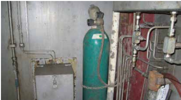
Temporary storage, secured with chain
