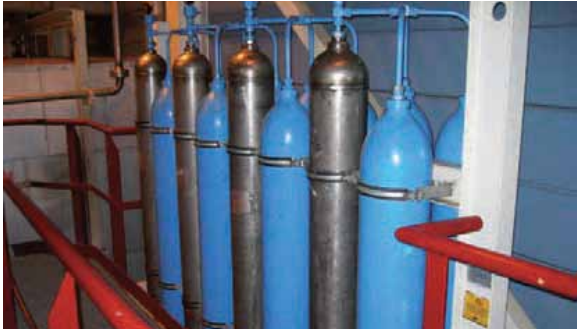
Storage rack with bolted cylinder brackets
