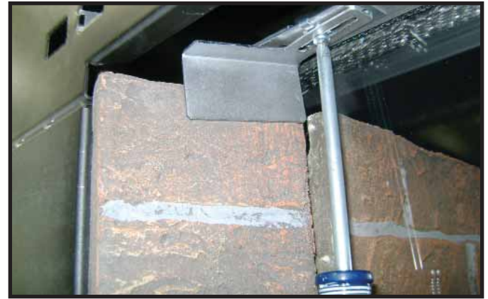
Figure 14.26 Side Refractory Brackets
