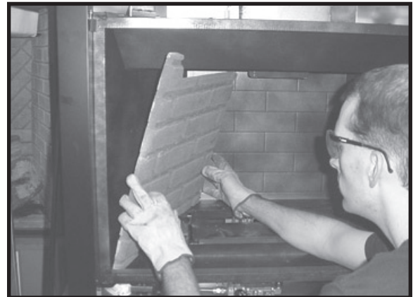
Figure 4 - Tip Side Refractory
