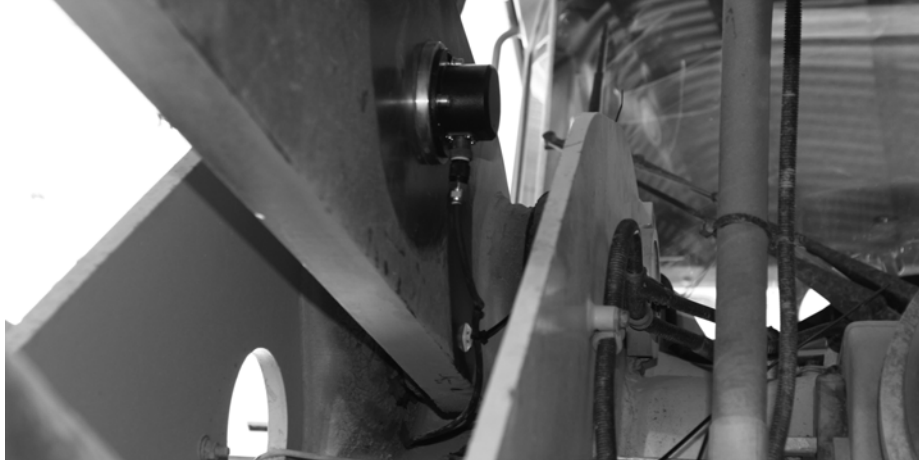
Figure 1-14. Angle Sensor Installed On Support Arm.
