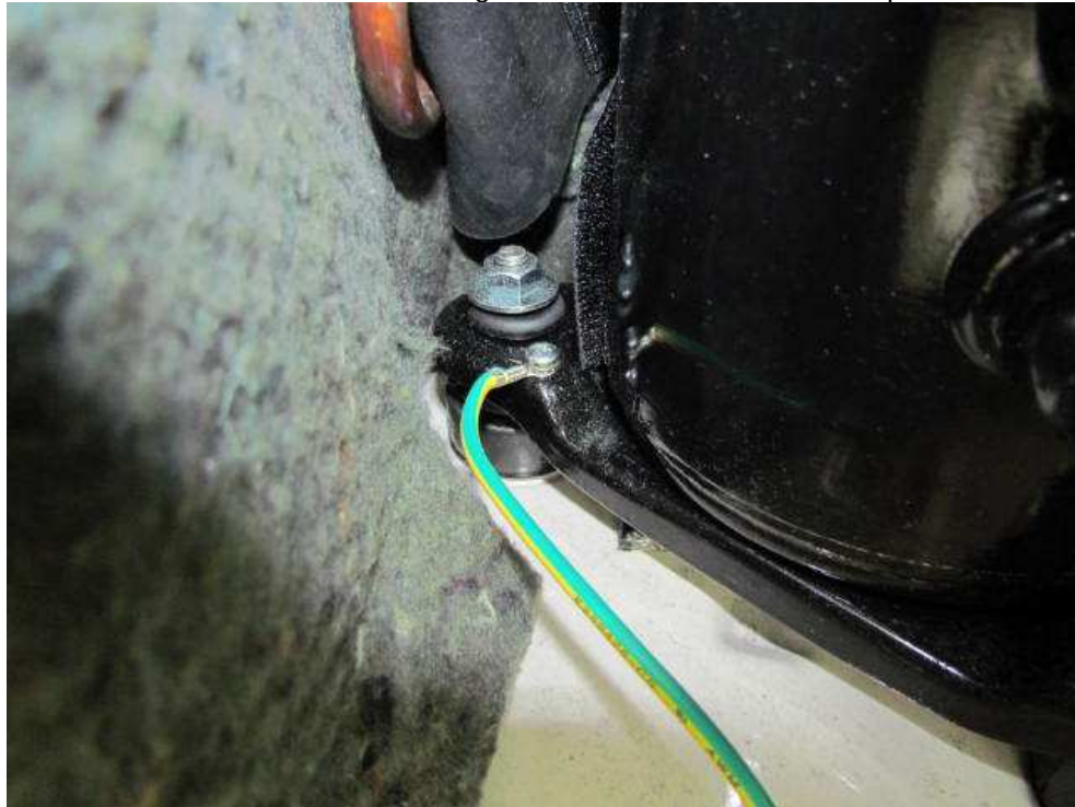
Earthing terminal block on compressor
