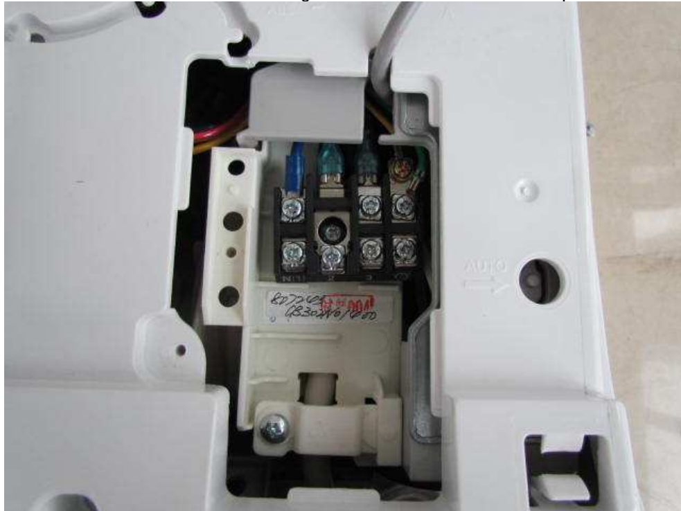
Terminal block view
