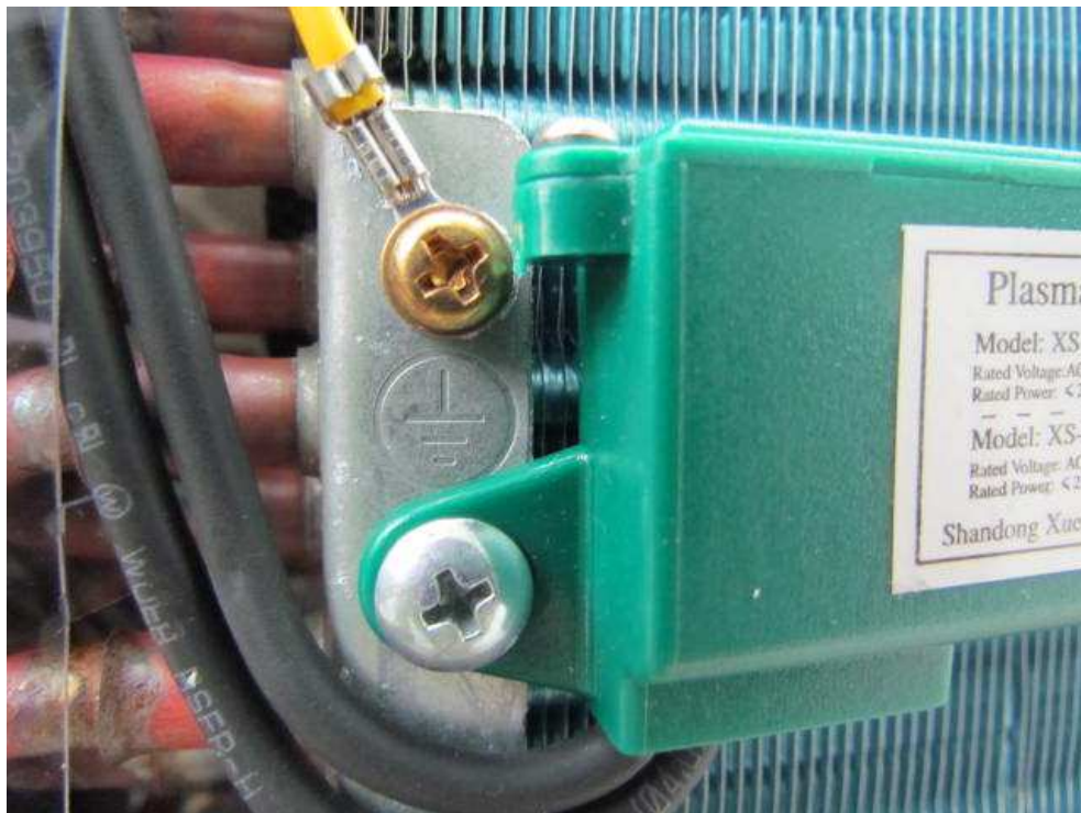
Earthing terminal on evaporator
