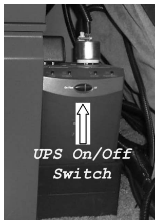
Figure 2.2.5.4. UPS on/off switch.
