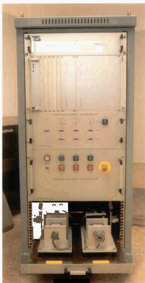
Fig. 4.1-1 TJS-TE general view
