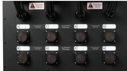
48 patch cables wired to eight 19 pin Socapex connectors labelled A thru H (6 circuits each) providing 48 outputs
