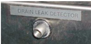
Figure 9-2: Pump Seal Drain Leak Detector Port
