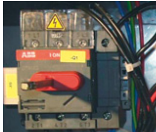
Figure 2-4: CryoPilot C Main Power Breaker
