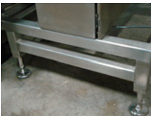
Figure 2-9: FT16 and Power Control Panel Leveling Feet
