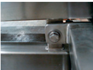
Figure 2-10: Power Control Panel Mounting Bolts
